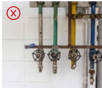
故障阀门和内漏位置，不易察觉 Hard to detect failing position or valves
